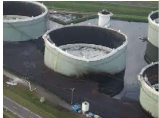
Crude Oil Storage Tank damage from roof collapse.
